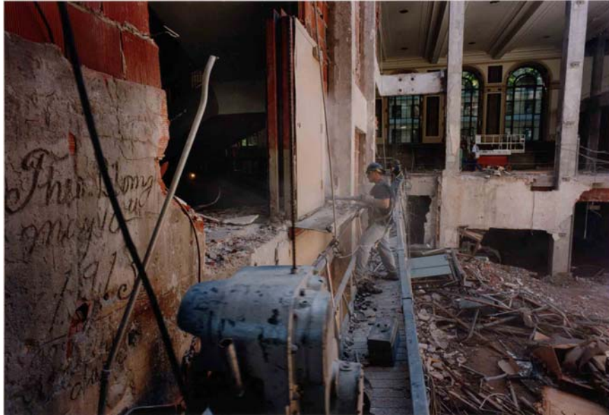
July, 1995 photograph of central library renovation project showing view into stack area. Note graffiti in plaster from original 1913 construction. From Department of Library Services Accession 2002-000293/018, Library Construction Project Records.
